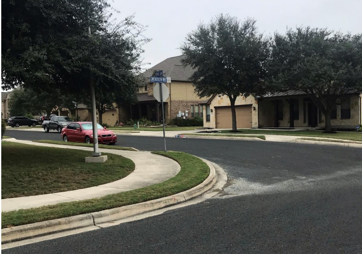
Figure 6- Severe chip loss at the corner of Gwendolyn Way and Hiram Lane
