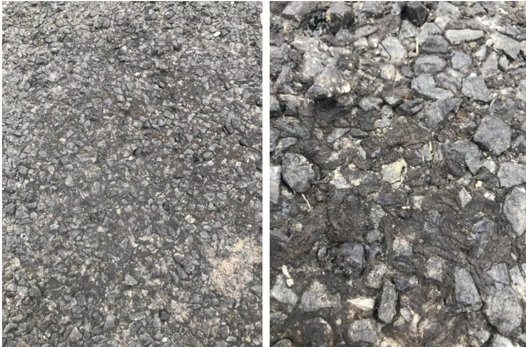
Figure 4- Excessive asphalt binder (Flushing) at cul-de-sac – Sophie Marie
